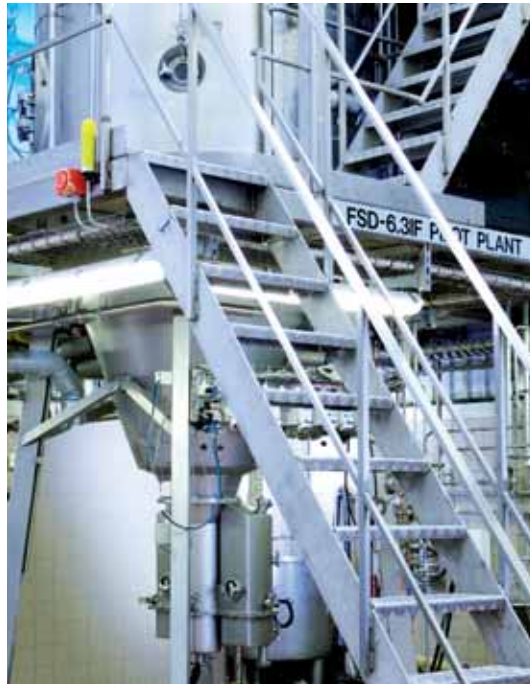
FSD™-6.3 with triple chamber static fluid bed. Installed in GEA Niro Test Center, Copenhagen. Drying chamber size: Ø 1600x800 mm, 40° cone.
